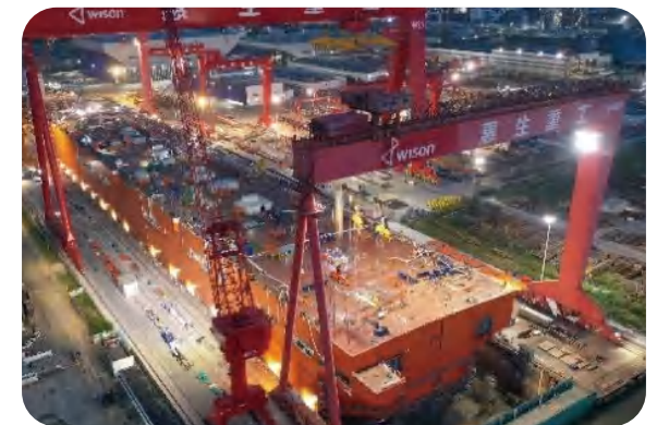
Main Deck Penetration of the NGUYA FLNG
